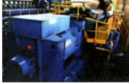
Combined Heat & Power
