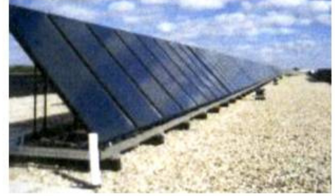
Solar Hot Water
